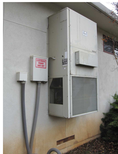
Figure 1: a classroom wall-pack HVAC unit.
